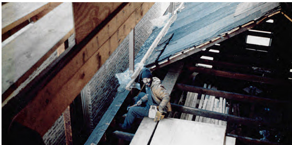
Bruno Ast (about 1975-76) working on renovation of 1756 Sedgwick. Visible is the existing former roof of building.
